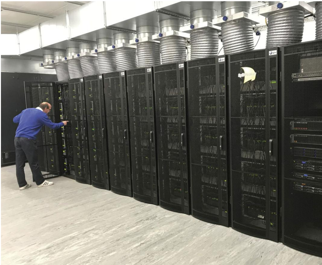
Figure 1: The million-core SpiNNaker machine at Manchester. The machine occupies 10 rack cabinets, each with 120 SpiNNaker boards, power supplies, cooling and network switches. The 11th cabinet on the right contains servers that support configuration software and remote access to the machine.
